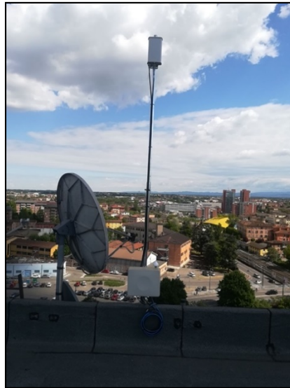
Figure 21. Photo of the installed antenna for the private cellular network used in CLASS
